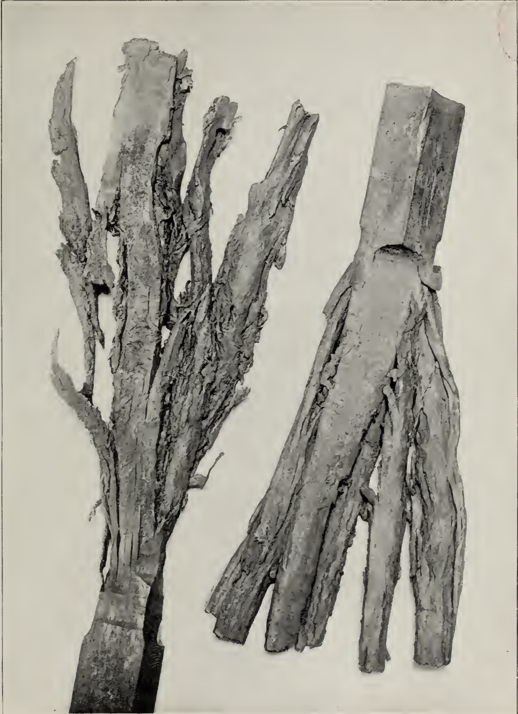
FIG. 62. DISINTEGRATED WROUGHT-IRON BARS
